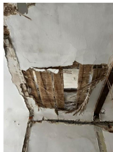
Fig. 4. Damaged ceiling over the ground floor (photo J. Markowska)
