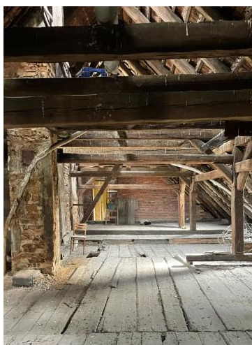
Fig. 6. Damage to the roof structure (photo J. Markowska)
