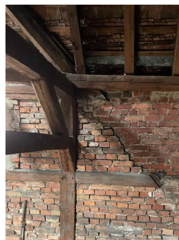
Fig. 7. A crack in the wall (photo J. Markowska)
