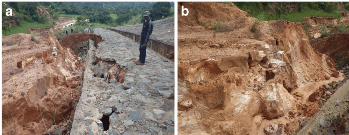
Fig. 4. Failure of prevention works due to instability in slope material [41]
