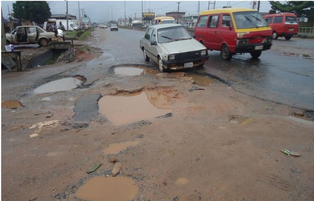
Fig. 3. Road failure aided by intense rainfall [36]
