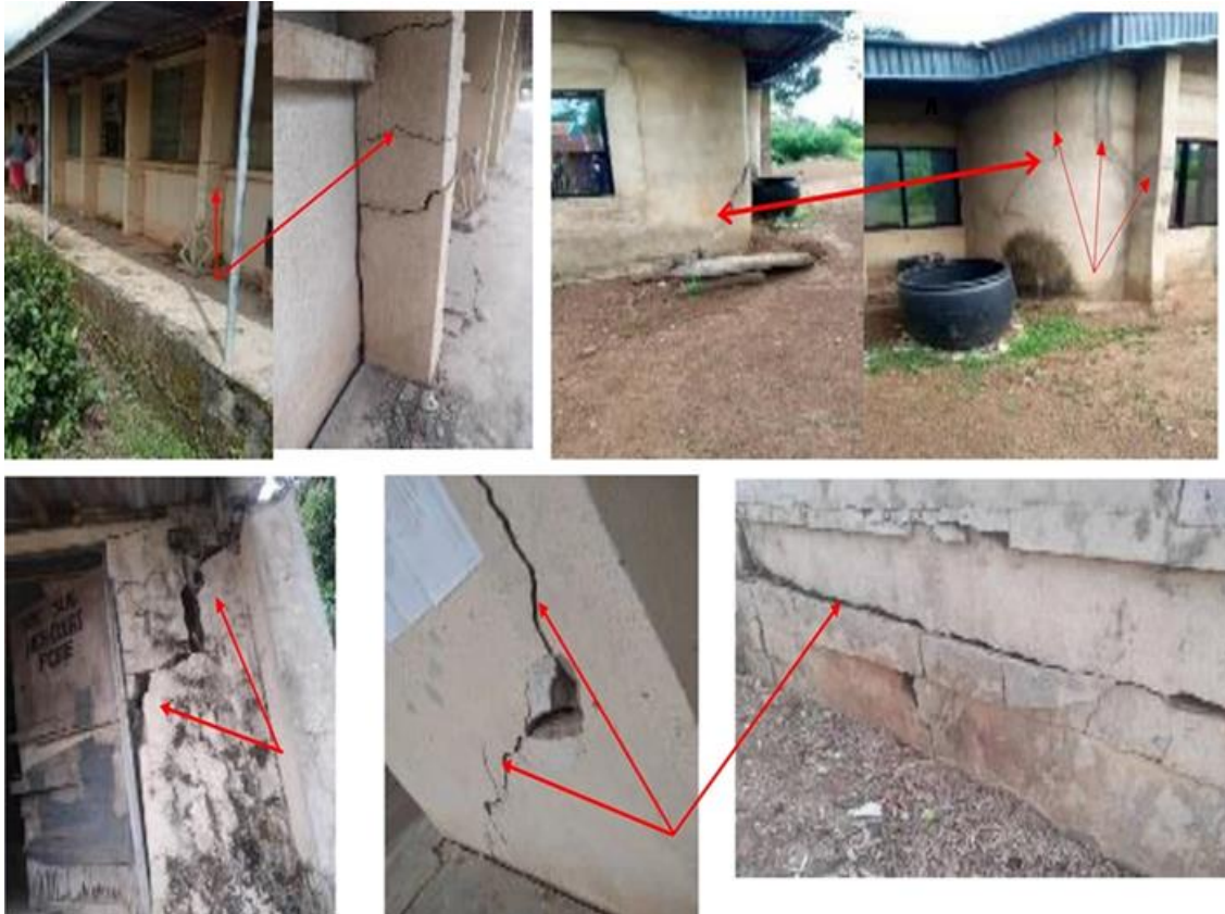
Fig. 2. Building foundation failures [3]
