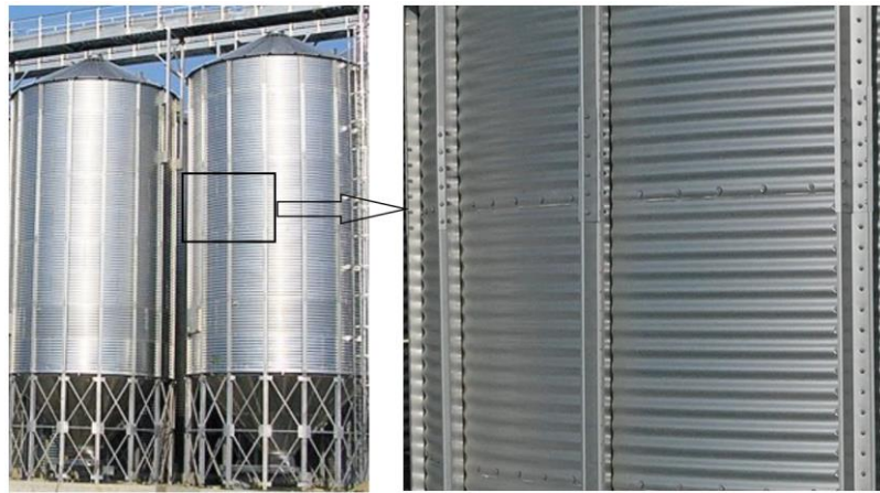
Fig. 1.1. Wall of a steel silo made of corrugated sheets strengthened by external stiffeners (ribs)
