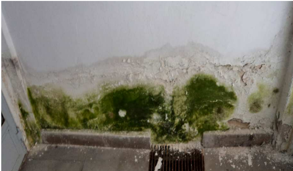
Photo 1. The external building wall with visible biocorrosion on the building of the former UZ canteen
