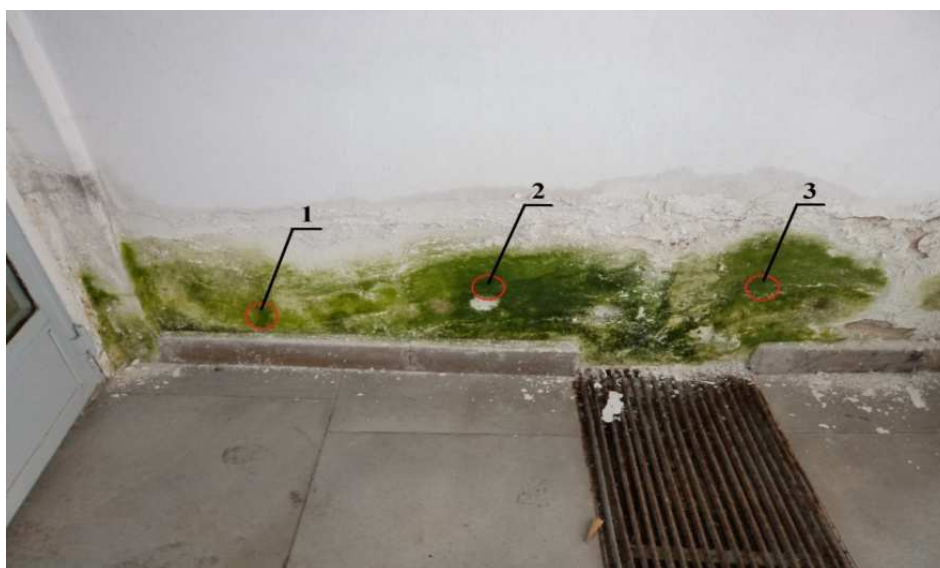
Photo 2. The three sampling points (marked 1,2,3) on the biodeteriorated external building wall
