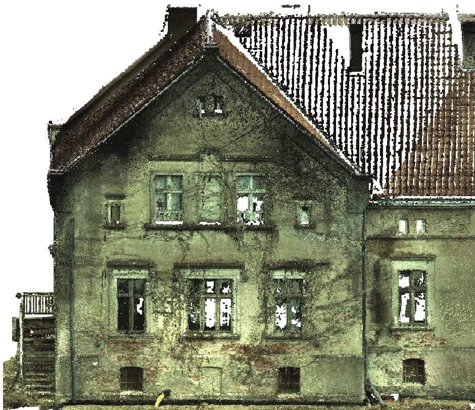
Fig. 4. Destroyed facade of a historic building (source: own study)
