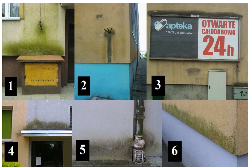
Fig. 1. View (1-6) on places in northern facades with visible discoloration and deposits
