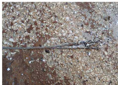
Fig. 7. Broken suspension line for radial scraper blades; aggregate in the bottom slab exposed as a result of excessive friction
