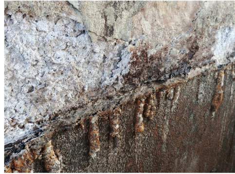
Fig. 3. Corroded concrete surface after detachment of the protective coating
