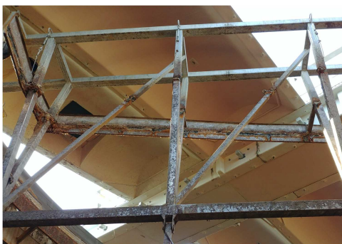
Fig. 6. Radial scraper lattice; visible strong concentration of steel element corrosion on the wastewater table level
