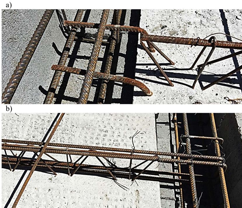
Fig. 6. Support reinforcement: a) rebars anchored from the top surface, b) U-type rebars
