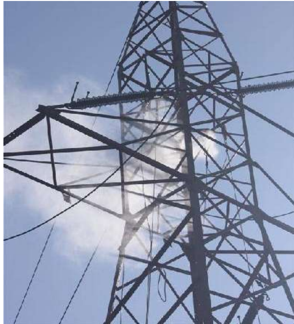
Fig. 4. Removing protective layers by sandblasting the steel pole of power line 400kV
