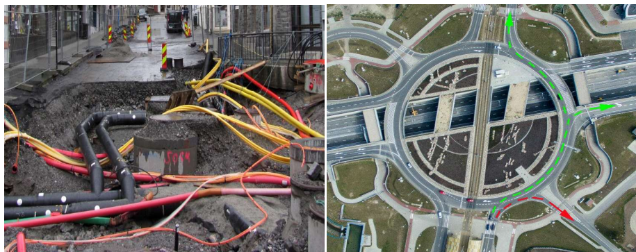
Fig. 13. Location of cables and pipes of underground integrated installations introduced into existing development [26]
