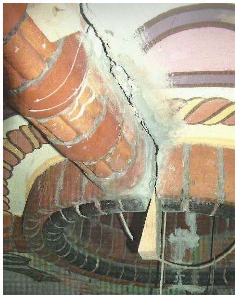
Fig. 9. Damaged area near the vault ribs and wood wedges driven in the place of cracking (2003)
