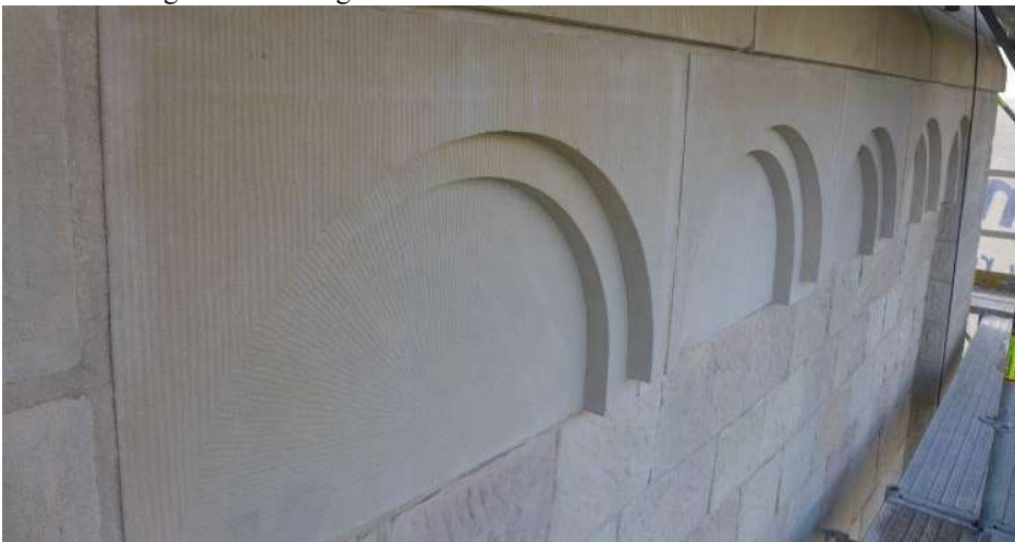
Fig. 22. Restored failure zone in the south tower
