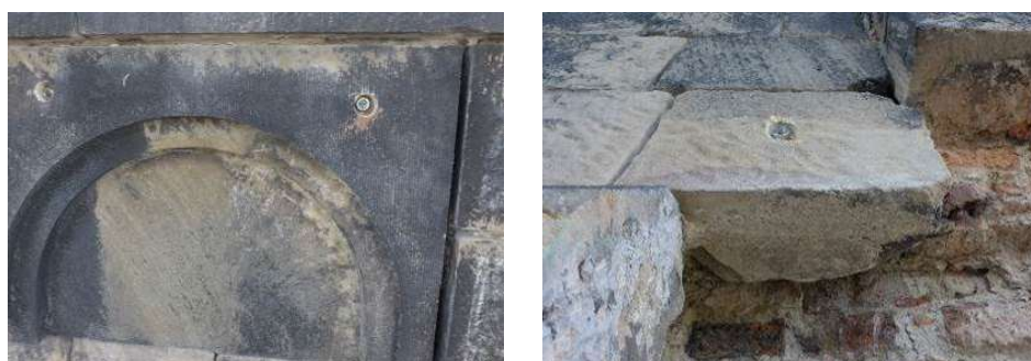
Fig. 19. Anchorage of loose elements
