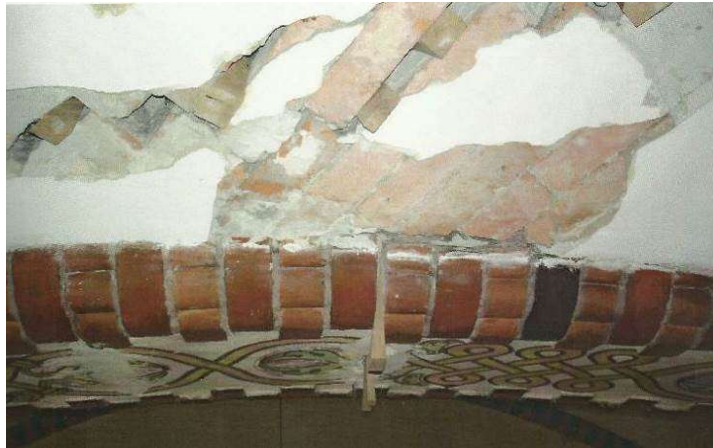
Fig. 8. Damage to the arch and wood wedges driven in the place of cracking (2003)
