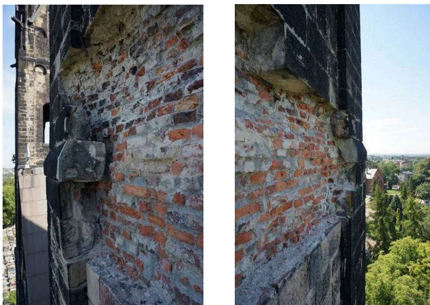
Fig. 12. Damage detail of the west elevation of the south tower
